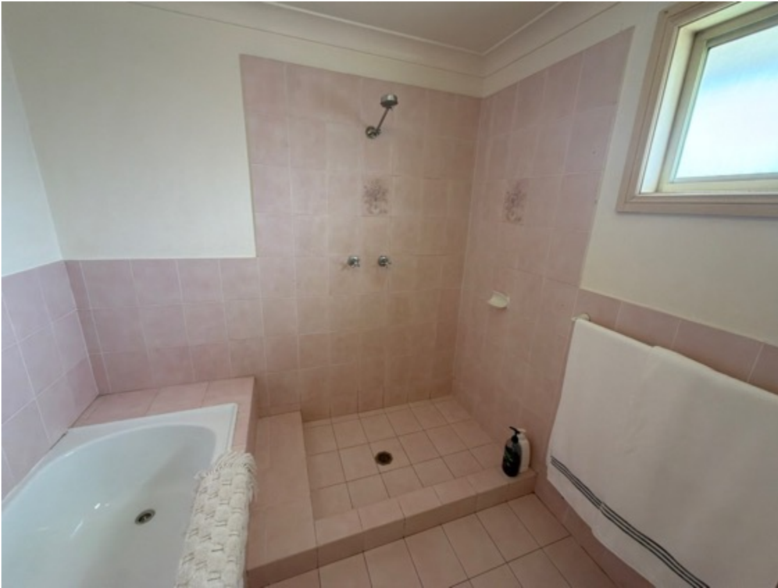
Water pressure tested, is sufficient.
