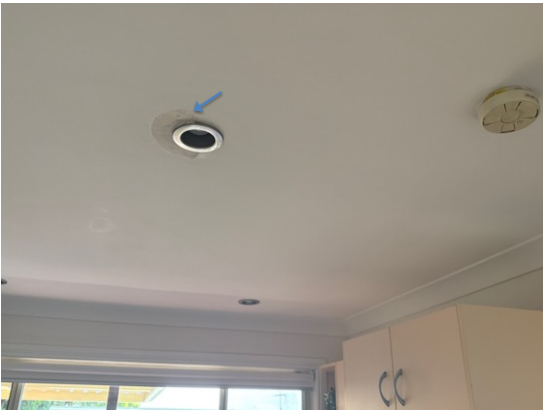
Patching around the ceiling light is incomplete.
