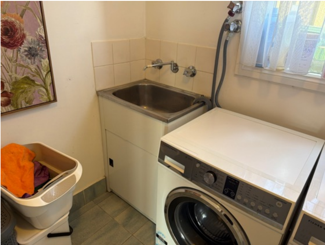
Water pressure tested, is sufficient.
