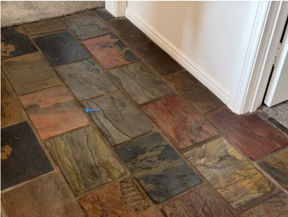
Isolated sections of internal tiles are chipped, consistent with age.
