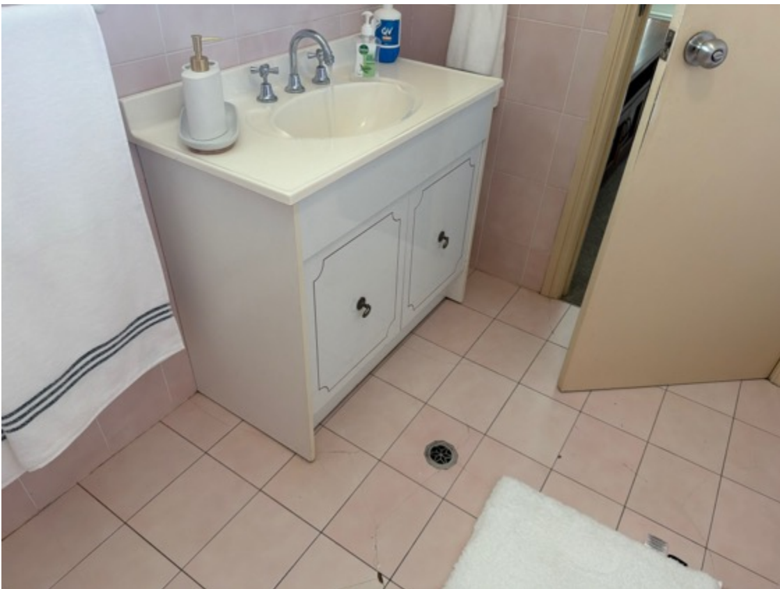
The vanity displays low level wear and sections of tiles are cracked, consistent with age.
