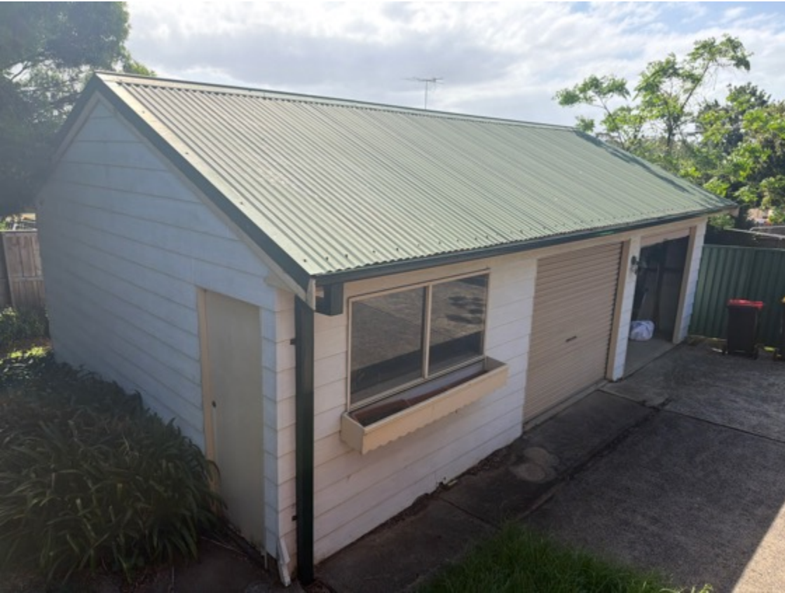
The shed is in serviceable condition for the age.
